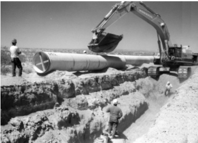
Construction of the Mojave River Pipeline to the greater Barstow area will deliver water to the recharge aquifer.
